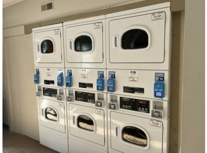
Subject's central laundry facility
